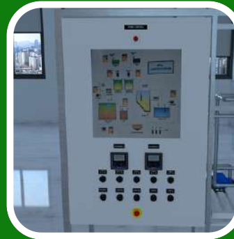
Kontrol Panel Digital (PLC)
